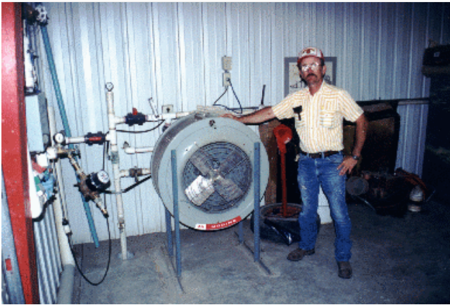
Figure 9. Modine heater in the Fire Station.
