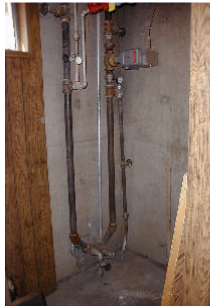
Figure 4. Two loops from the DHE entering the home—one for space heating and the other for domestic hot water.
