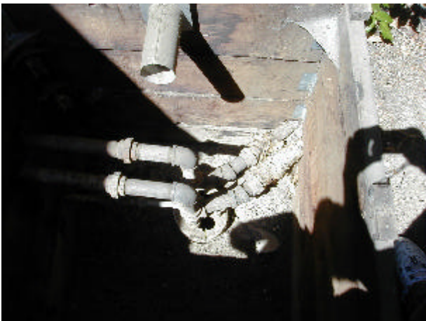
Figure 2. Well with three DHEs, a single 2-inch (5-cm) pipe used for space heating and two 3/4-inch (2-cm) pipes used for domestic hot water.
