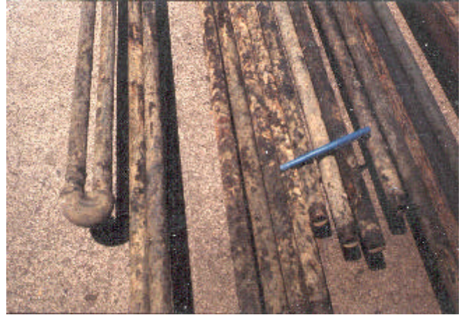
Figure 3. Corrosion and pitting of DHE replaced in 1974. Note the reverse loop at the bottom of the heat exchanger.
