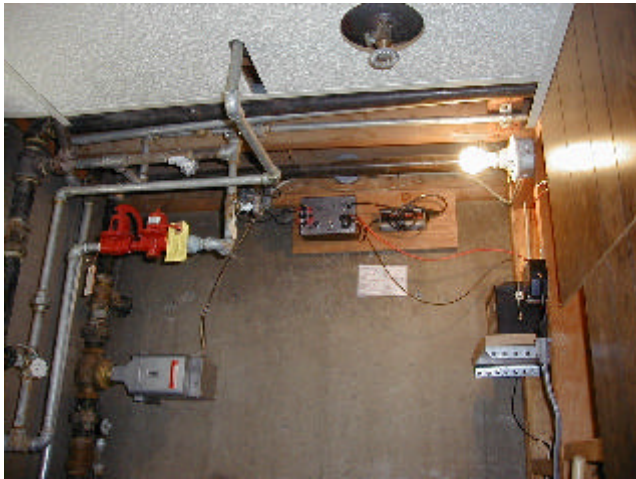
Figure 5. Motorized control valve, solid state controller and expansion tank - the pressure reducing and pressure relief valves in the foreground.
