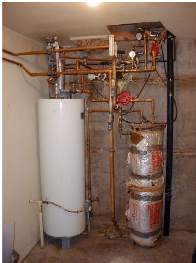
Figure 8. The interior mechanical system showing the domestic hot water shell-and-tube heat exchanger on the right and the water storage tank on the left. The pipes from the DHE enter at the top-center of the photograph. Circulation pumps can also be seen in the center top.
