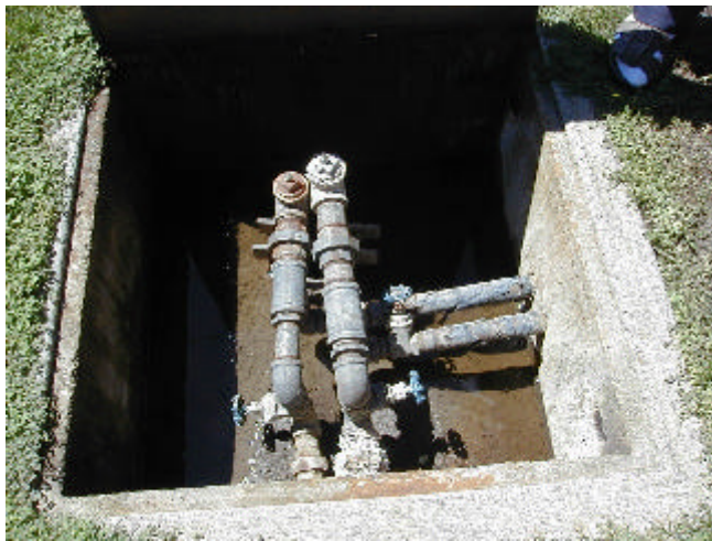
Figure 7. Well head with a single DHE and two supply lines.
