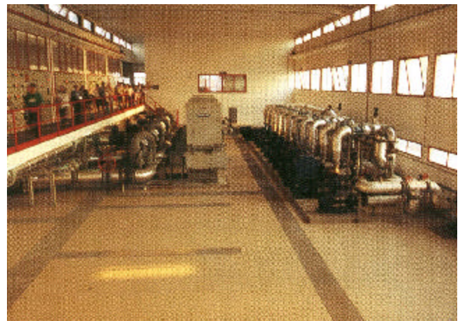
Figure 5. Ferrara pumping plant.
