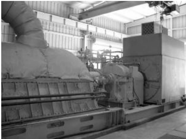
Figure 10. The condensing turbine.
