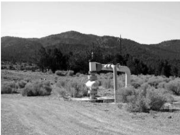
Figure 6. Photo of the CFSU 42-7 wellhead.
