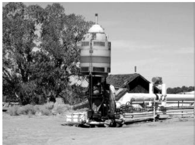
Figure 7. Photograph of well P91-4. The well is equipped with a pump.
