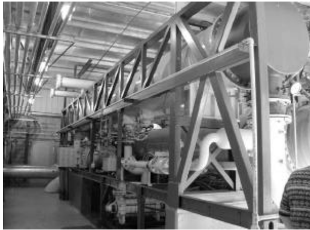
Figure 9. One of the ORMAT binary units.
