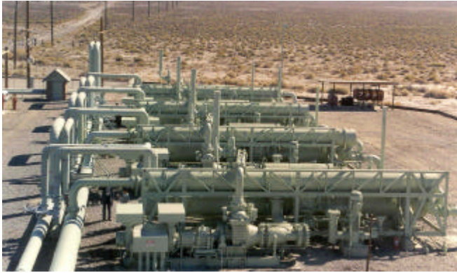
Figure 7. Binary power plant in Empire, Nevada.
