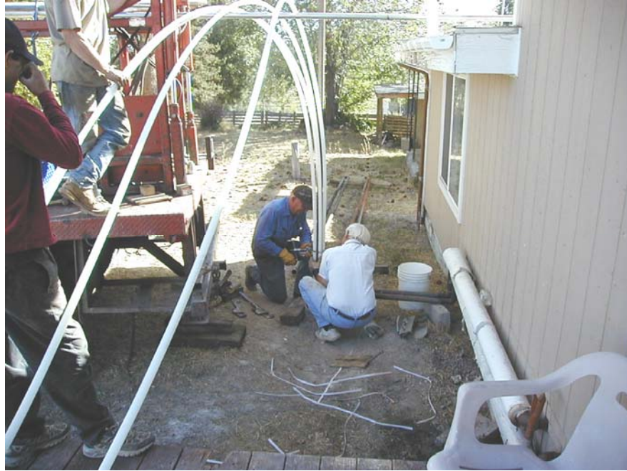
Figure 4. PEX DHE prior to installation, showing the two PEX U-tubes fastened to the black iron pipe of the old DHE, which was used as an installation guide, anchor, and convection promoter.
